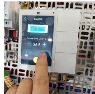
Fig. 14: HVAC control by using smart touch panel
